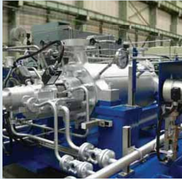
Ring Section Boiler Feed Pump Qurayyah CCPP Saudi Arabia, 5x266MW
