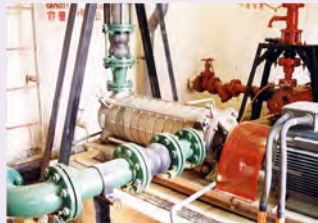
Stainless-steel feed pump for building facility
