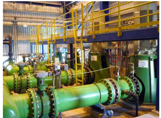
Make up Water Pumps
