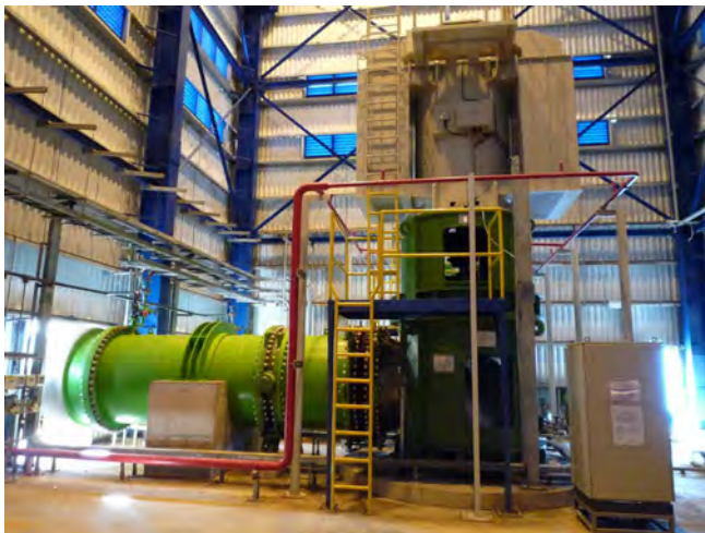
Main Cooling Water Pumps
