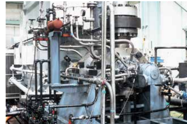
Fujairah Combined Cycle Power Plant, 3 x 660MW, U.A.E. MHG ring section boiler feed pump
