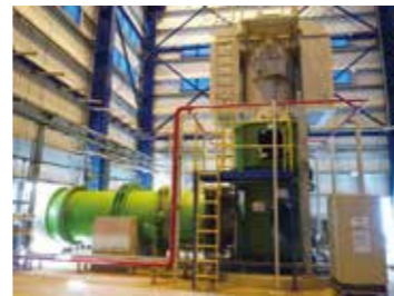
Balance of Plant (BOP) for the pumping facility of power plants
