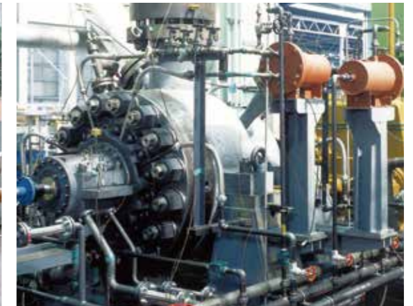
Elbistan B Coal Fired Power Plant 4 x 360MW, Turkey MHB barrel type boiler feed pump [12.6MW drive, 100% duty]
