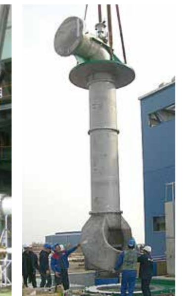
Germencik Geothermal Power Plant 45MW, Turkey CDKTV hot well pump
