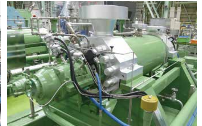
Keys Energy Center Combined Cycle Power Plant, 1 x 755MW, U.S.A. MHG ring section boiler feed pump
