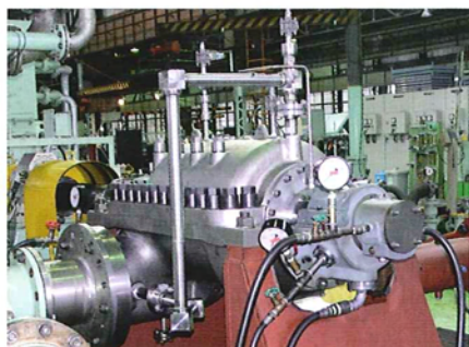
Shuwaikh RO Project (Kuwait), 2009 ;— MHH200/4 704m 3 /h at 660m 1800kW
