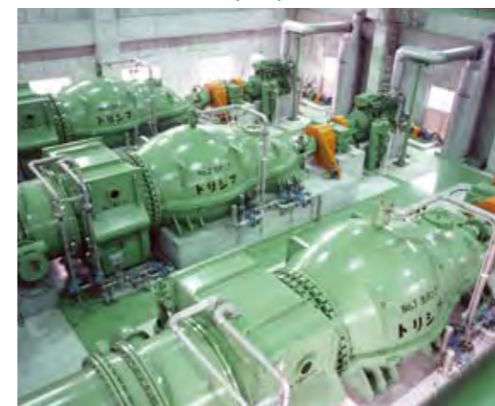
[Horizontal mixed-flow pumps]
