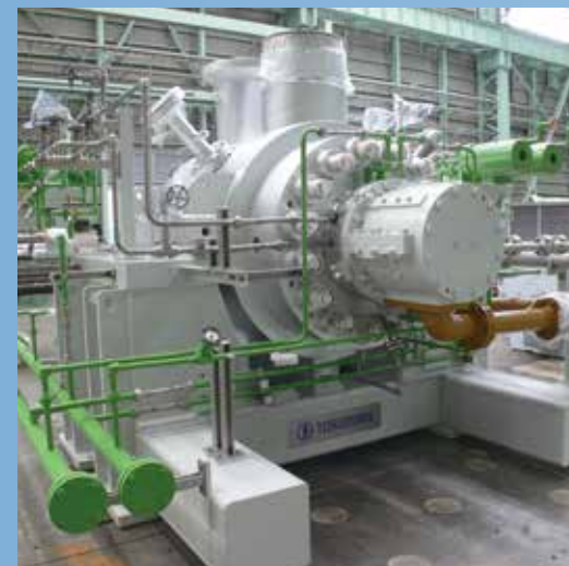
Barrel Type Boiler Feed Pump Chhabra Supercritical Coal Fired PP India, 2x660MW
