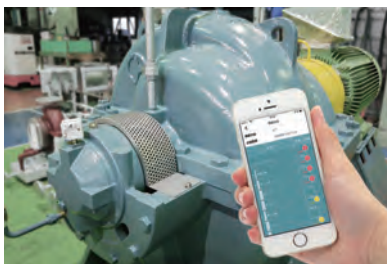
Maintenance and inspection (monitoring of machine conditions)
