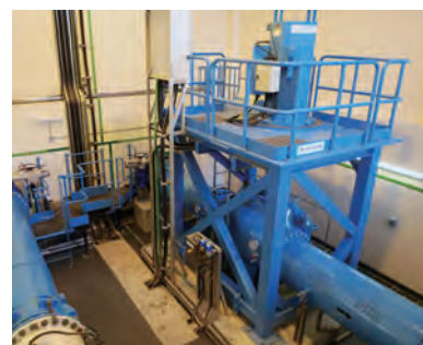
Vertical-shaft reverse-rotated pump turbines
