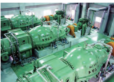
Irrigation pumping stations
