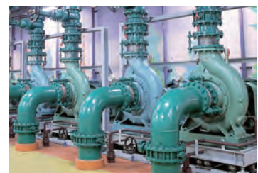
Cooling water pumps for district heating and cooling facilities
