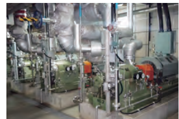
Boiler feed pumps for incineration plants
