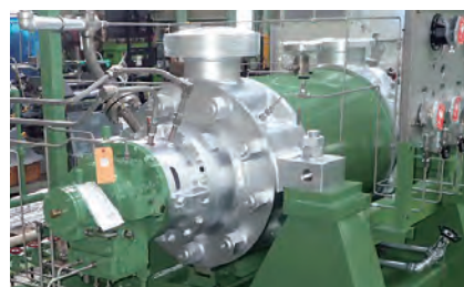
Boiler feed pumps for biomass power plants
