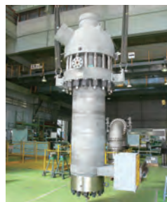
Boiler circulation pumps
