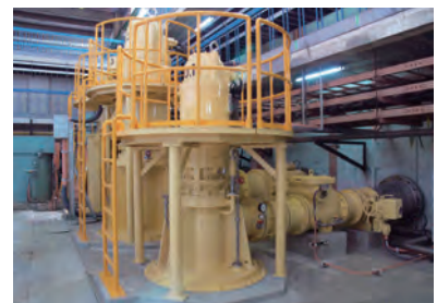
Pump facilities at sewage treatment plants
