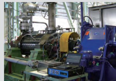
Performance test of boiler feed pump
