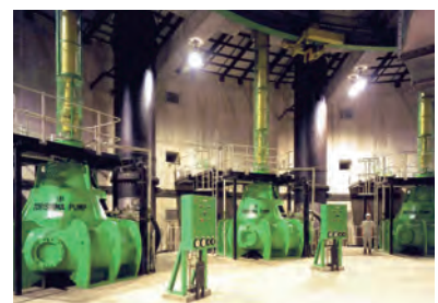
Sewage relay pumping stations
