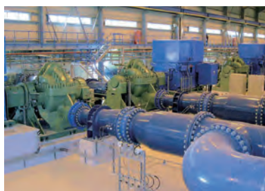
Long-distance water transmission pumping stations
