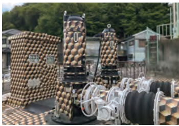
Supplying pumps with submersible motors (Disaster prevention and mitigation)
