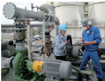
Energy conservation diagnosis of pump facilities
