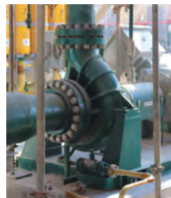
ERD pressurized pumps
