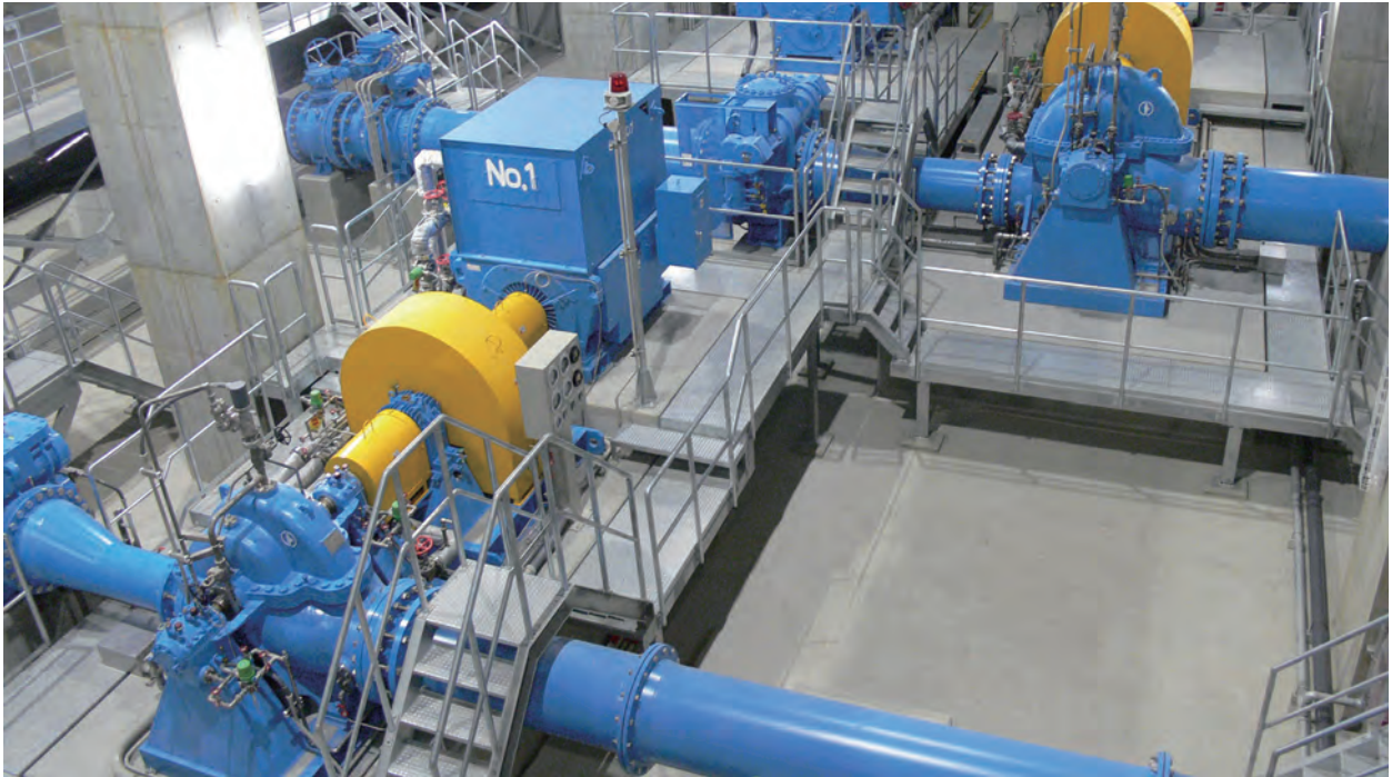
Water transmission pumping stations
