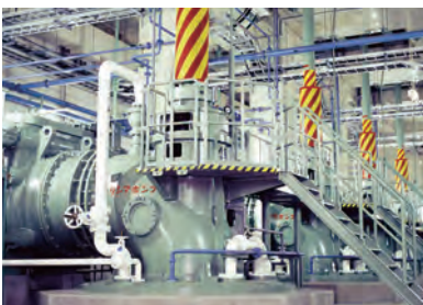
Stormwater drainage pumping stations
