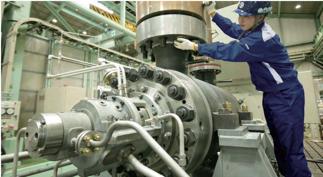
Boiler feed pumps (Barrel type)
