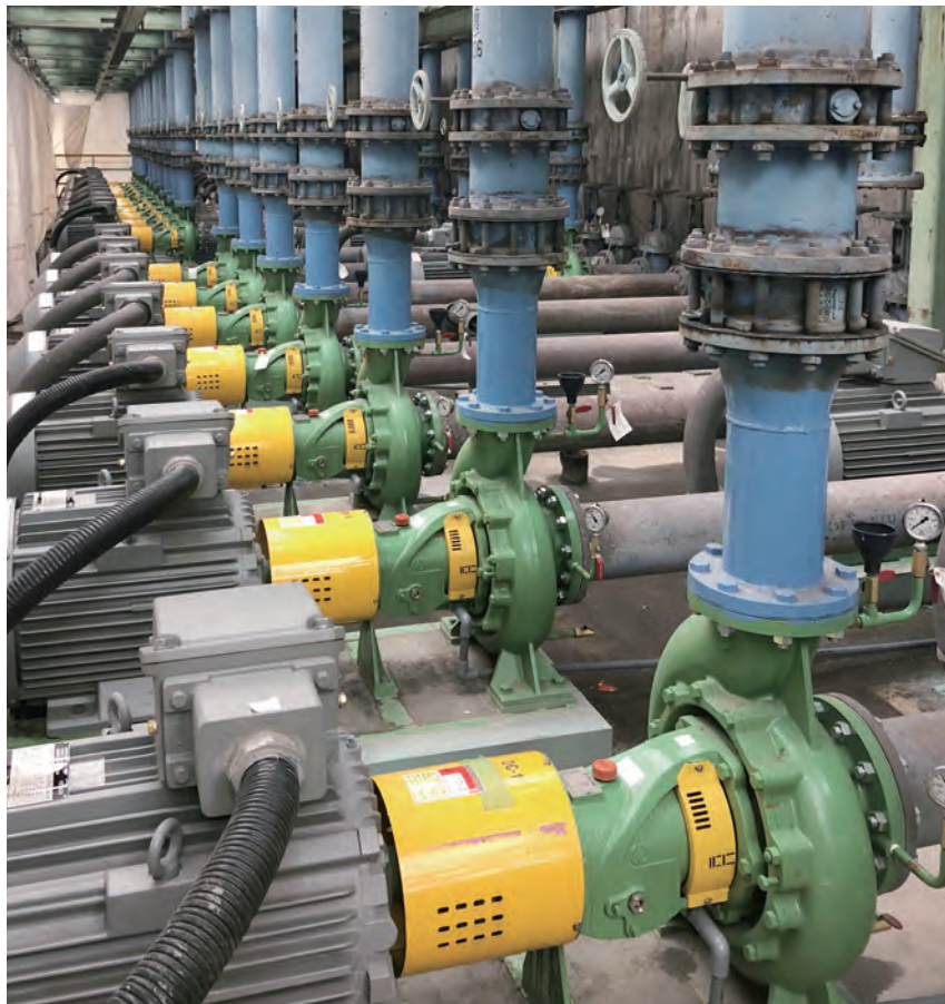
Cooling water pumps for electric furnace manufacturers
