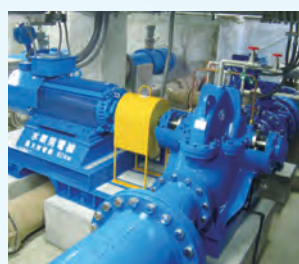
Reverse-rotated pump turbines
