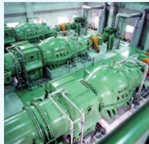
Irrigation pumping stations
