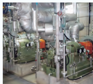
Boiler feed pumps for incineration plants
