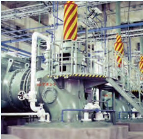
Stormwater drainage pumping stations
