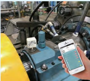
Maintenance and inspection (monitoring of machine conditions)
