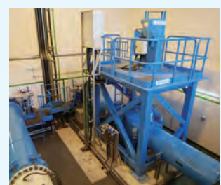
Vertical-shaft reverse-rotated pump turbines
