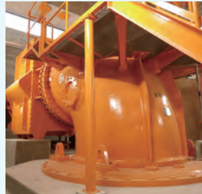
River drainage pumping stations
