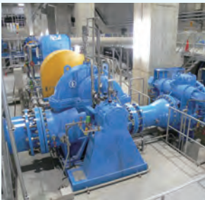
Water transmission pumping stations
