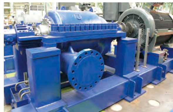
Reverse-osmosis high-pressure pump
