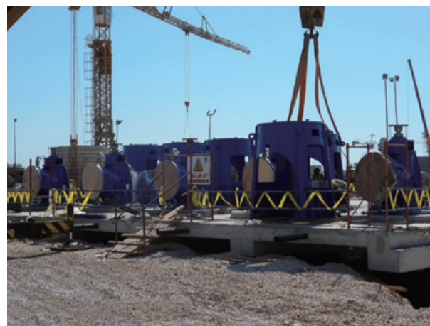
Torishima water treatment pumps being installed at the Bahr Al-Baqar Treatment Plant
