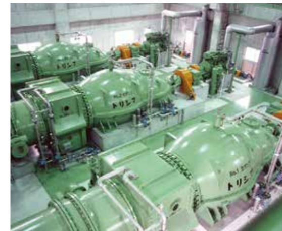
[Horizontal mixed-flow pumps]
