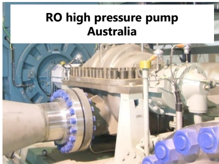
RO high pressure pump Barren
