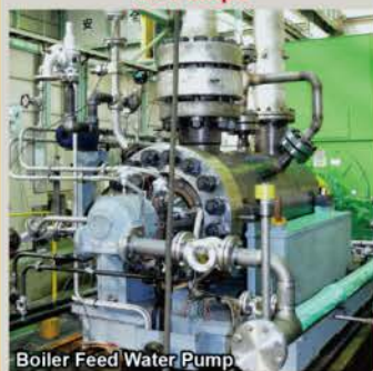
Boiler Feed Water Pump
