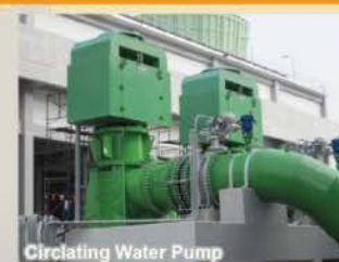
Circulating Water Pump
