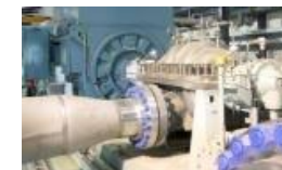
2007 High pressure seawater supply pump for RO desalination
