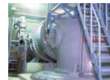
1981 Ultra-large drainage pump facility in Kyushu, Japan
