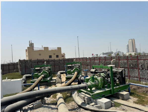
Pump station - Ras Al Khor Wildlife Sanctuary
