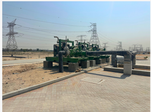
Pump station - Nad Al Sheba
