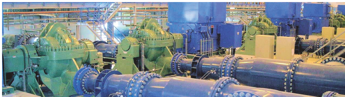
Potable water transmission pump, Size : 800mm × 500mm, 250m - 79m 3 /min - 4700kW
