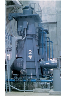
Water distributing pumps Size : 700mm 48m - 60m 3 /min - 650kW
